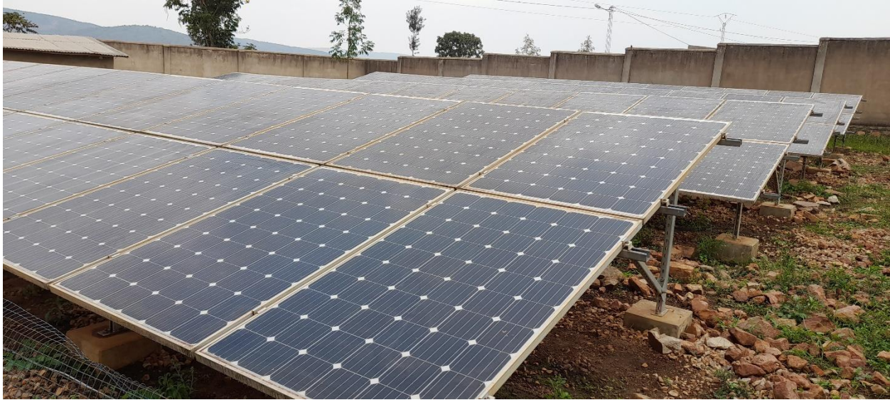
Photo 6 Solar panels of the “dead system” at the RDC premises that was resurrected
