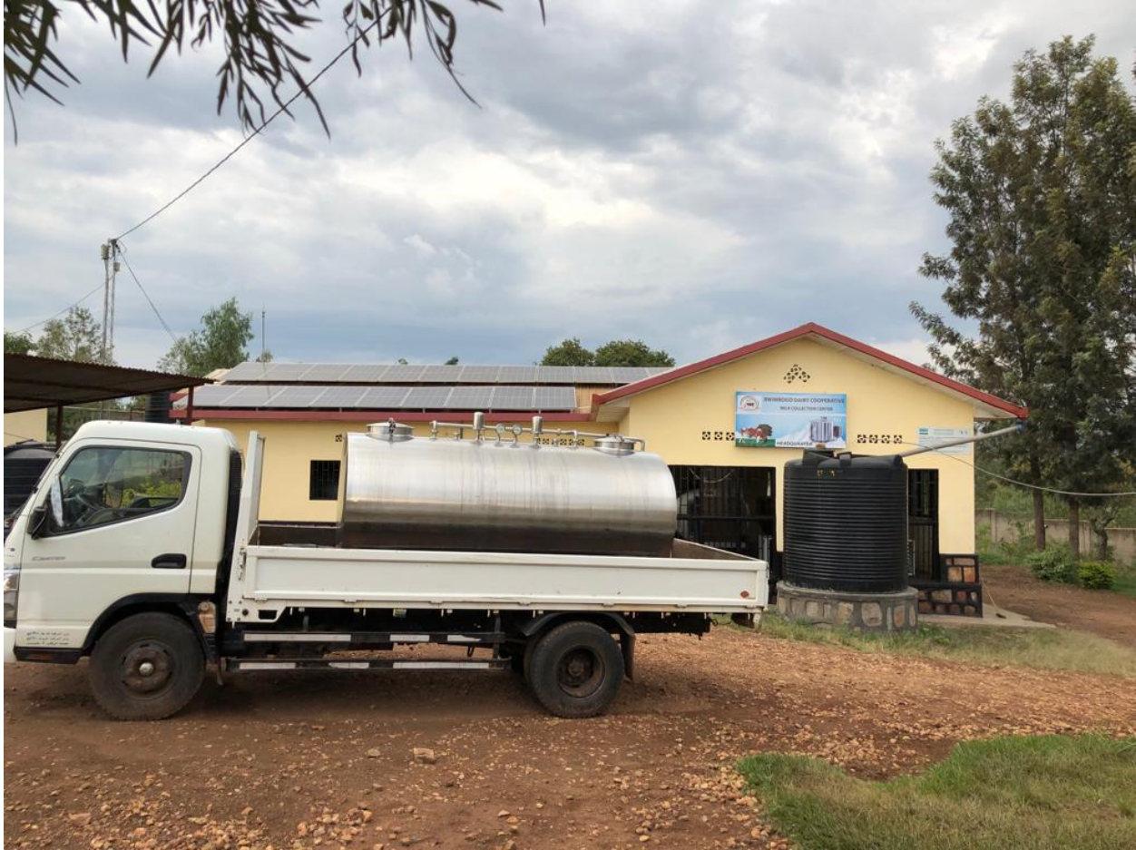
Photo 7 Additional solar panels that were installed by CET on the rooftop of the MCC
