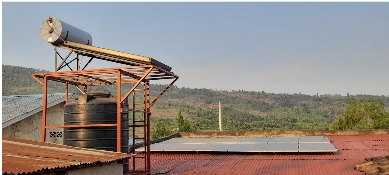
Photo 4 Solar panels and solar hot water installed at the RDC MCP in Rwagitima trading center
