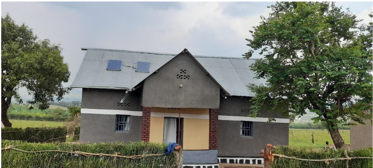
Photo 8 Two 120 W solar panels installed on top of the roof of the house of Joyce Mushmirwa to power her
