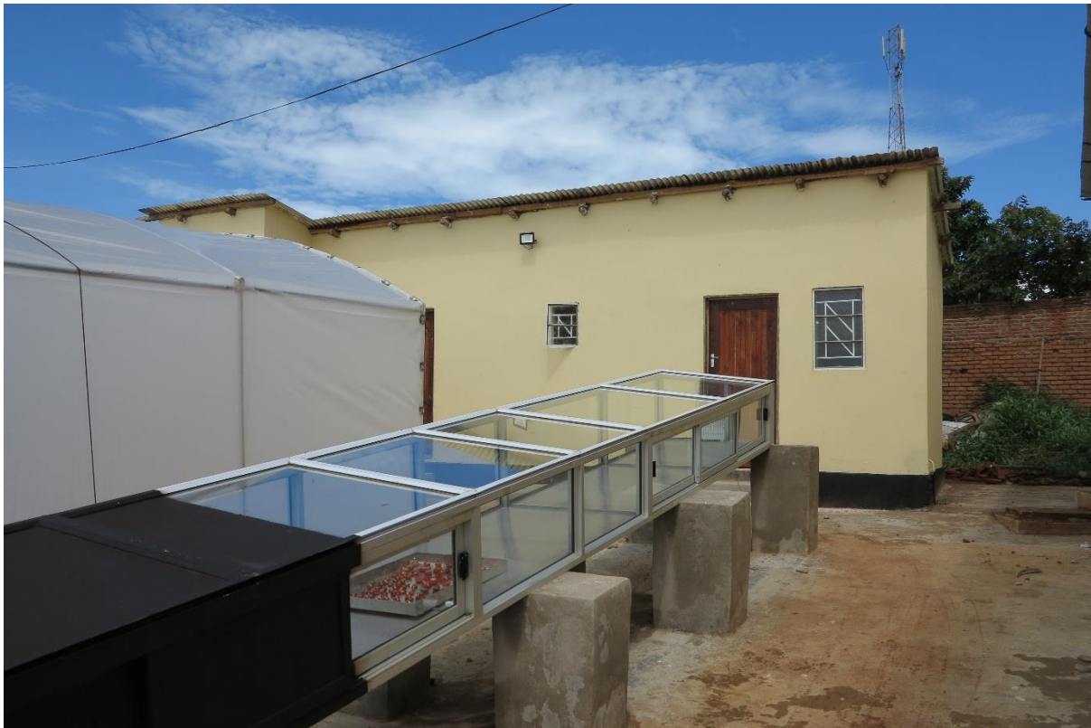
Pack house adjacent to the dryers – solar panels are on the roof and batteries are in the building.
