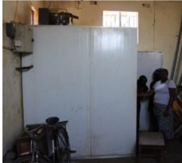
Figure 6: Cold room not in use inside Chia Fish Market building, Nkhotakota
